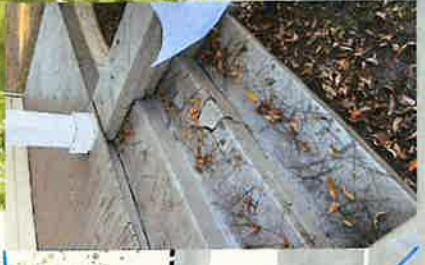
EXISTING FRONT STAIRS AND DECKING CONDITION
