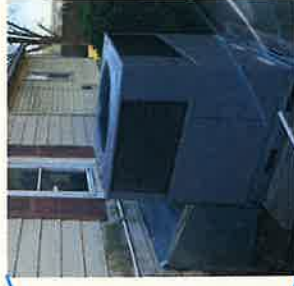
EXISTING MECHANICAL EQUIPMENT
